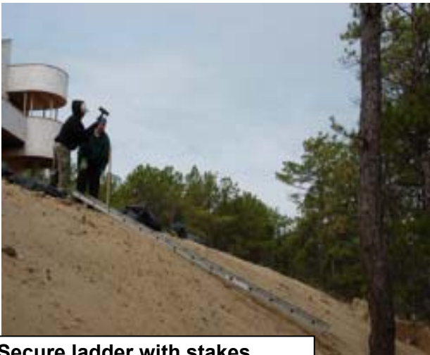
Secure ladder with stakes
