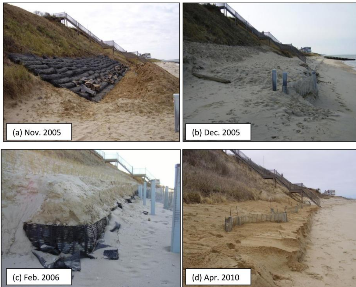
Figure 10 – View of a marine mattress with gabion toe coastal engineering structure permitted and installed at 28 Hinckley Lane, Nantucket (a) during construction, (b) after construction, (c) following coastal storm erosion, and (d) after annual nourishment to re-cover the marine mattress and gabion toe structure.
