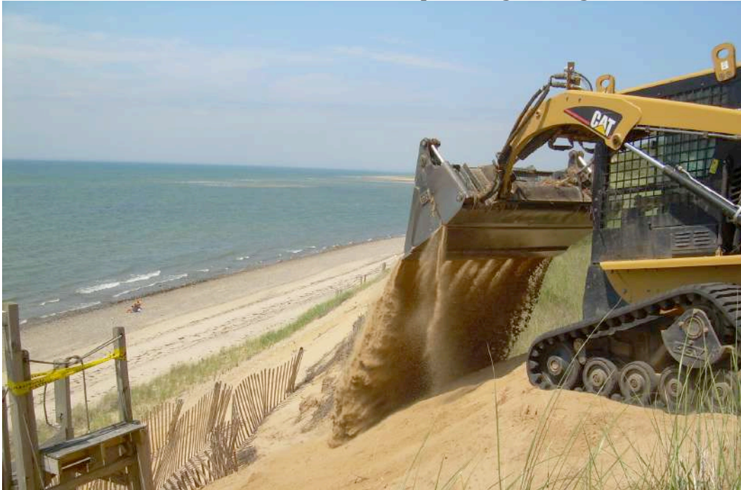
Image by G. Peabody: Over bank renourishment can be spot directed using small equipment. This project utilizes sand from on site excavation materials
