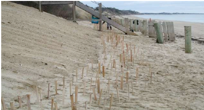
Biomimicry sand collection system at toe of nourishment area.
