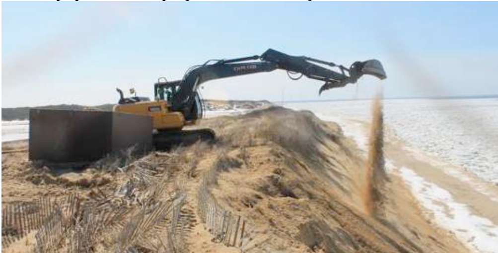
Safe Harbor Image above shows “full bank” nourishment. Sand is delivered to dump box from sand storage area. Equipment transfers nourishment along the full height of the bank, providing longer term, more sustainable, bank protection
